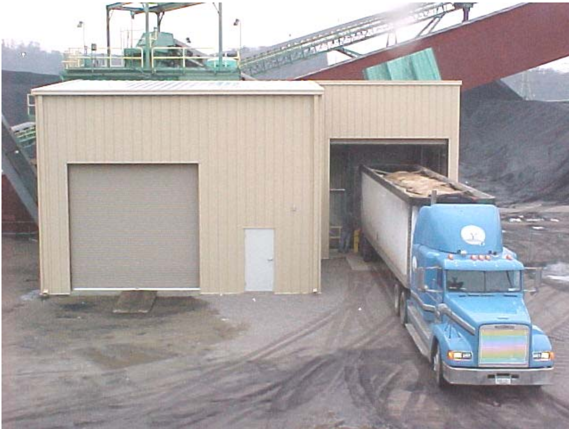
Figure 2. Cofiring Installation at Willow Island Generating Station. This Installation Includes Fuel Receiving, Screening, and Grinding of Oversized Particles in the Main Building (shown), and Fuel Storage, Reclaim, and Metering (to the main belt) in the Walking Floor Bin (not shown).
