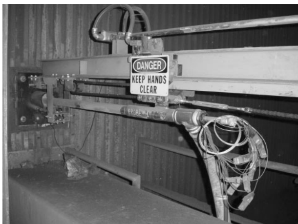
1 Corrosion probe installed at mid-western utility
